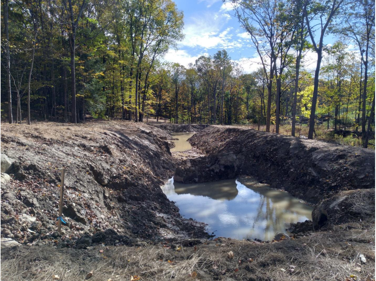
First pond constructed, seeded, and mulched. Pond has not yet filled with water.
